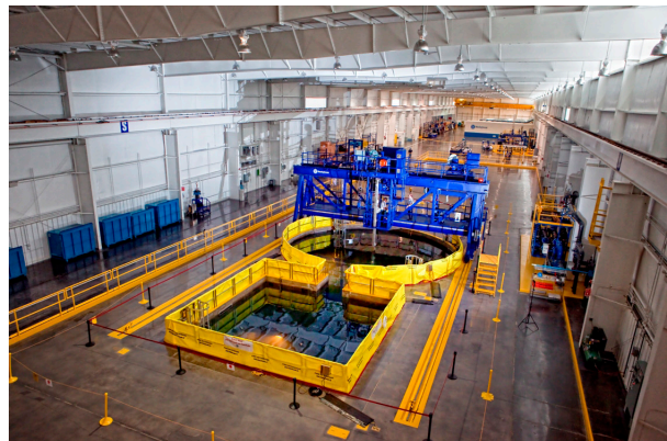
Westinghouse's BWR Service Center features a full-scale BWR cavity with vessel, internals, SFP and refueling bridge, two 33-ton cranes and an under-vessel mockup.
