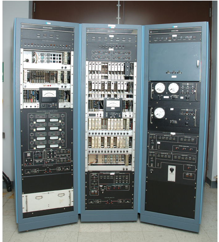
BWR nuclear instrumentation system training equipment located at Westinghouse Waltz Mill facility
