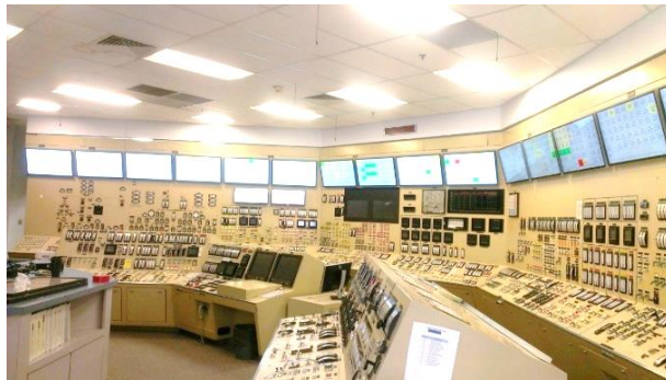
Annunciator Replacement in Westinghouse SNUPPS Simulator
